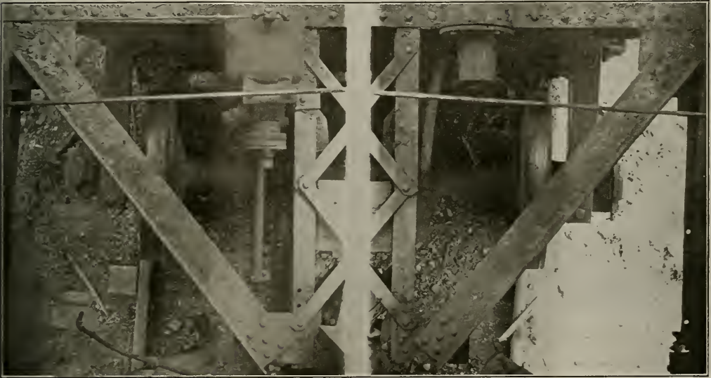
UNINJURED DIAGONAL BRACE IN CAR WITH BROKEN END.
